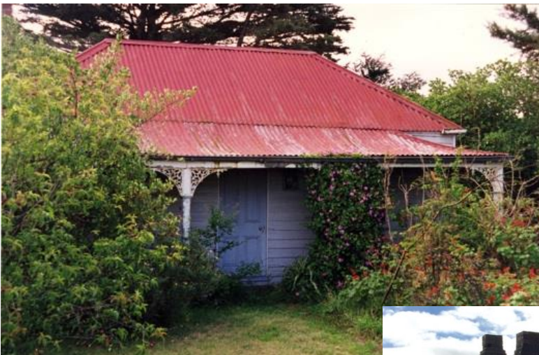
John and Mary Hurley's house on the Glencairn property at Ceres. Left: in 1998. Below: in 2016 Photos: Euan McGillivray
